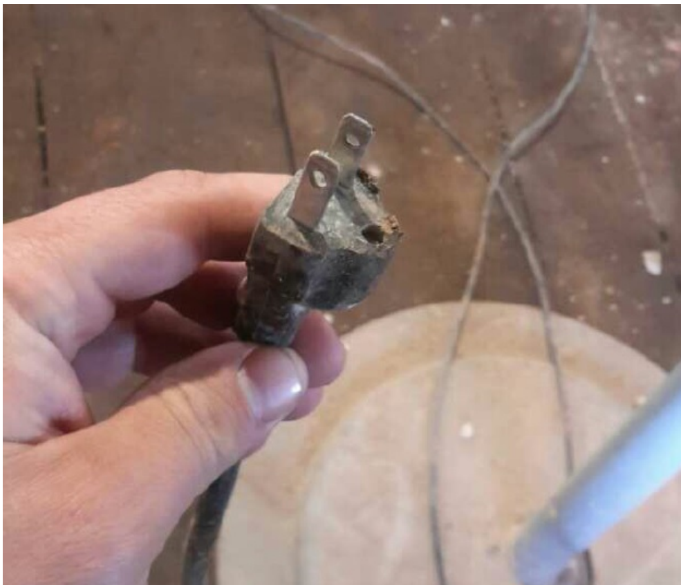
Inspect Extension Cords Prior to Use. No Grounding Pin, Do Not Use The Cord.
